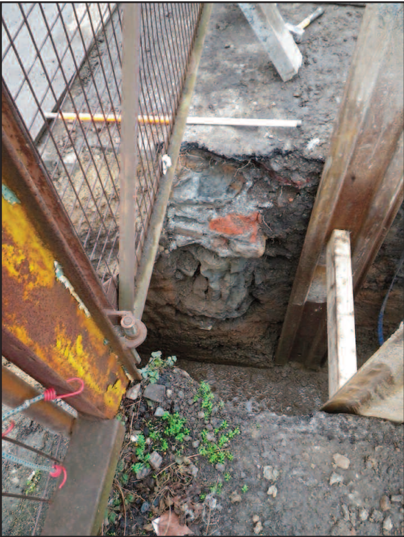
Plate 3 Wall 103 in the service trench at the southern boundary of site, looking north-west
